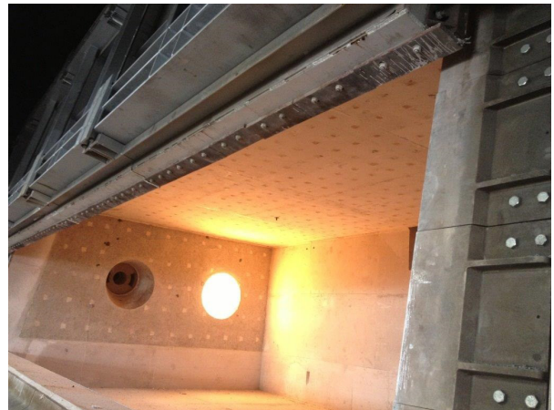
Furnace lined by Pyrotek's TAB Refractory Services.
