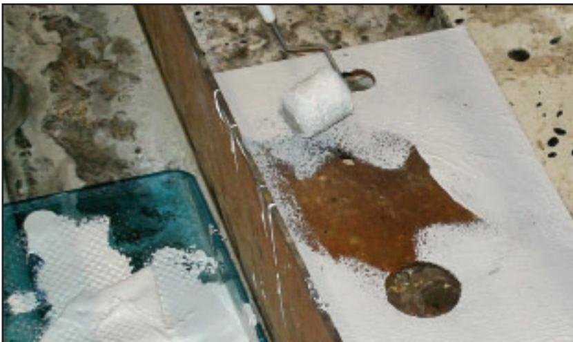
Exposed and rusty metal on the casting deck represents an extreme risk for molten metal explosion. Proper application of Wise Chem reduces the risk of serious personal injury and plant damage.
